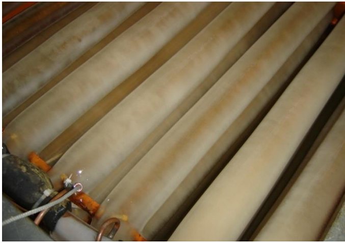
FIGURE 3. Ice cylinders formed around the evaporator coil during a test.
